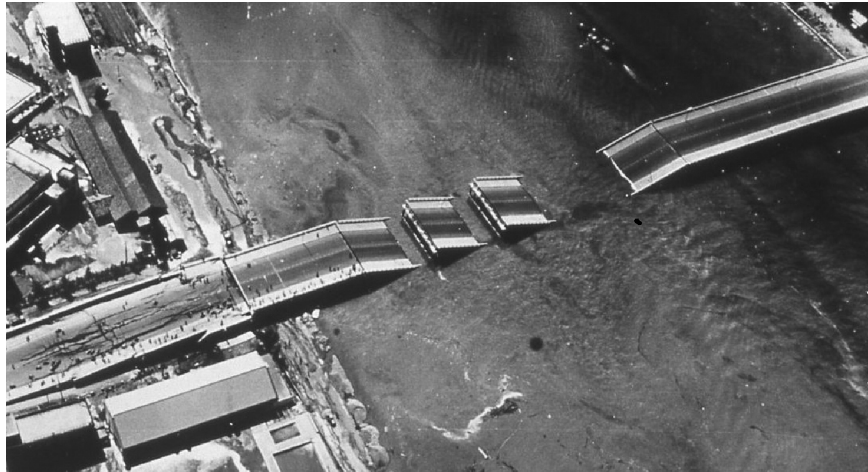
Figure 3. Showa Bridge failure due to 1964 Niigata earthquake and liquefaction phenomenon (Kerciku et al 2008) [13].
