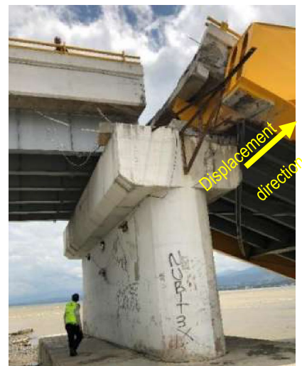
Figure 2. Bridge support failed due to earthquake (Budiharto, 2021) [12].
