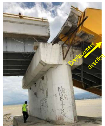
Figure 2. Bridge support failed due to earthquake (Budiharto, 2021) [12].
