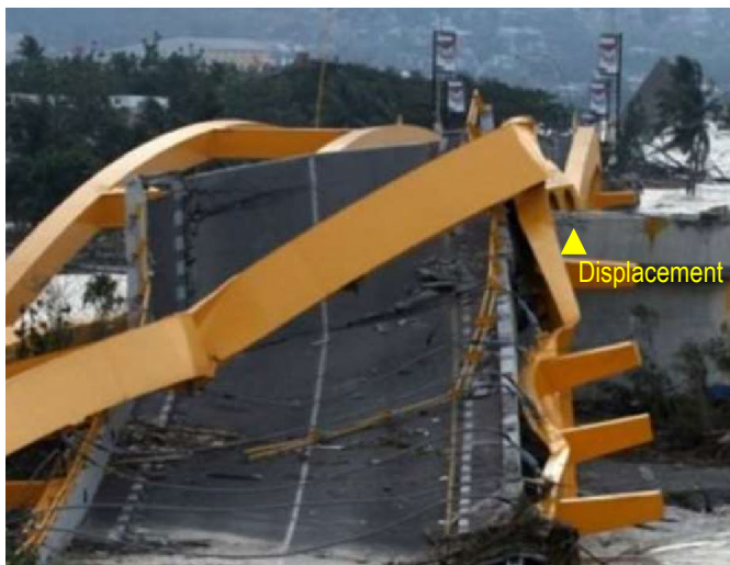
Figure 1. Palu IV Bridge has collapsed after Palu Earthquake 2018 (Nurdin, 2021) [11].
